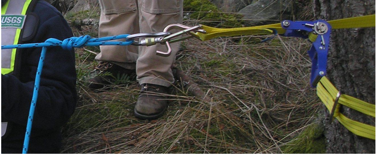
Figure 5. Span rope is connected by a carabineer to the come-along, which is secured around a tree.
