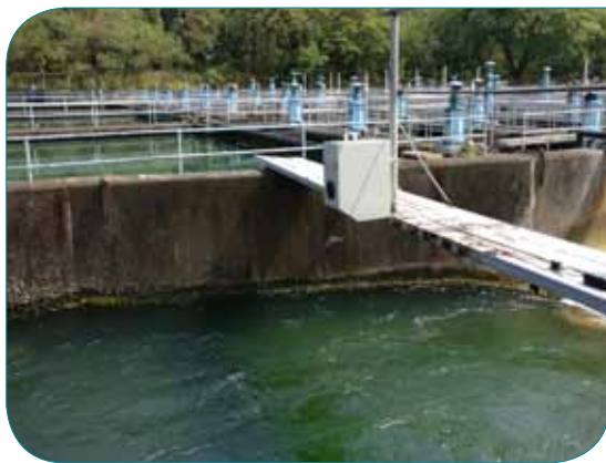
Pic: Installation of RQ-ADMS in the water treatment plant
