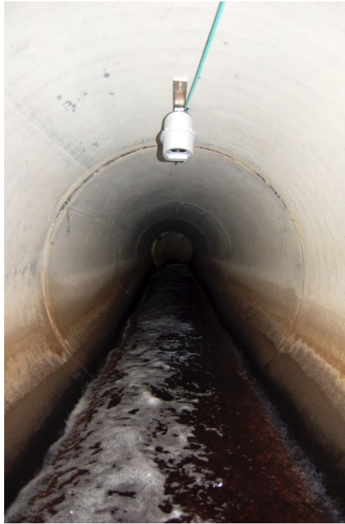
Figure 10 Installation of a SQ-R sensor in a water discharge channel
